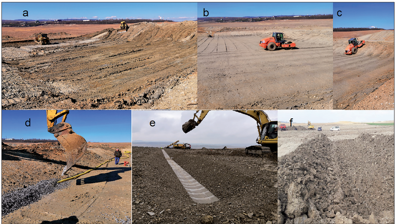
Fig. 4 Key steps of catchment construction a) excavation, b,c) construction of sealing, d) construction of drainage system, e) detail of surface runoff collecting ditch, f) overall view on finished array.
